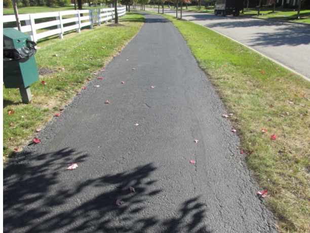
Edge cracks at asphalt pavement walking path
