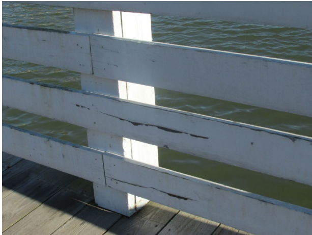
Wood deterioration at railing
