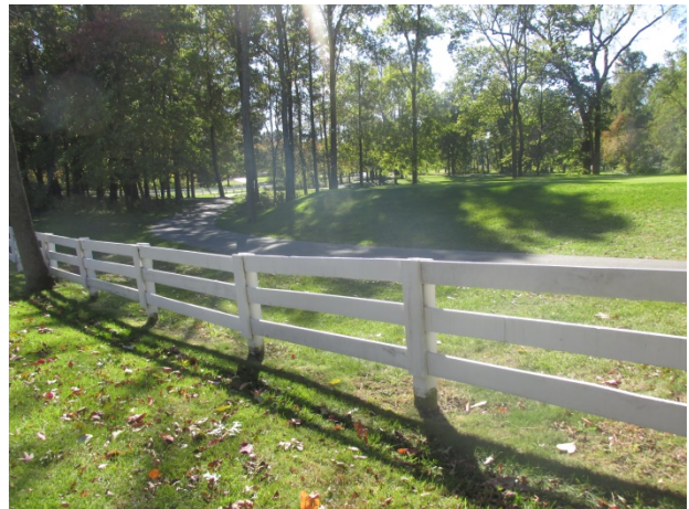
Wood fence with isolated deterioration at base of post
