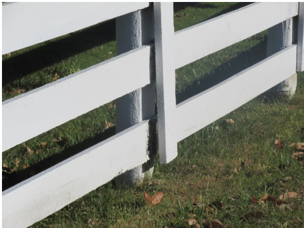
Loose post at wood fence
