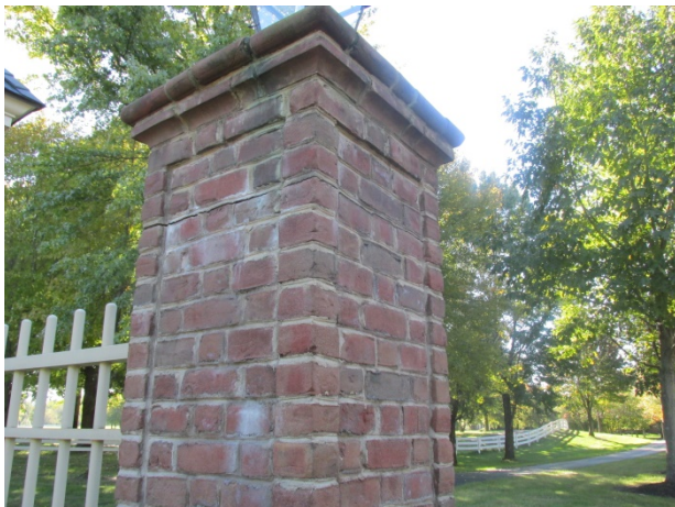
Efflorescence at masonry monument
