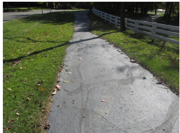
Cracks at asphalt pavement walking path
