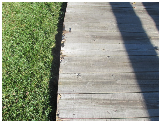
Isolated deck board deterioration
