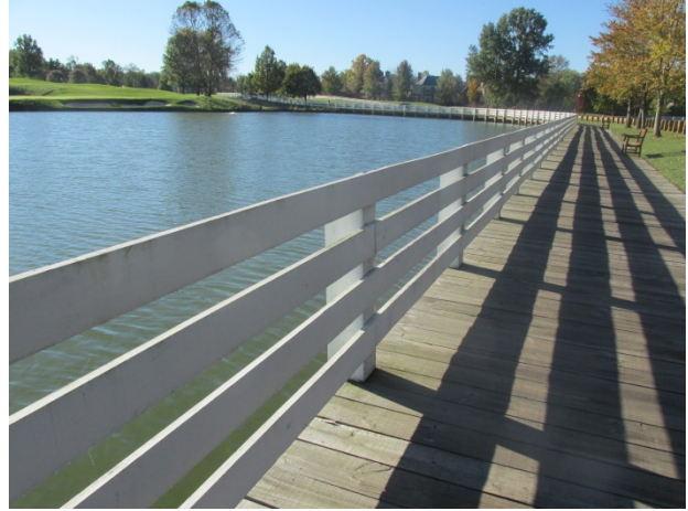
Railings at boardwalk
