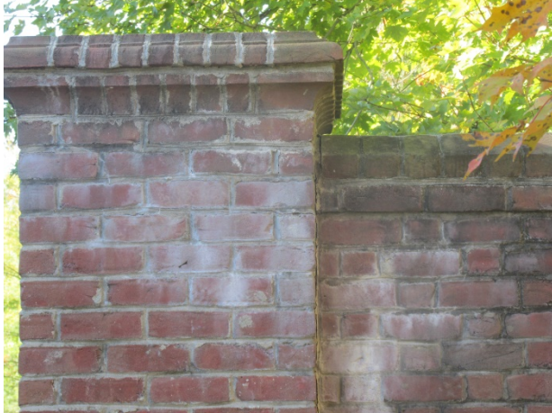
Efflorescence at masonry monument
