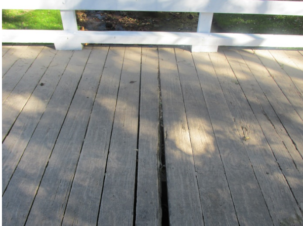
Wood deterioration at bridge deck boards
