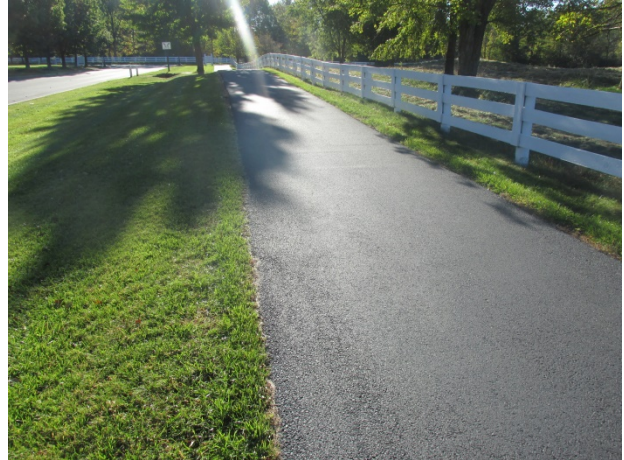
Previously replaced asphalt pavement walking path
