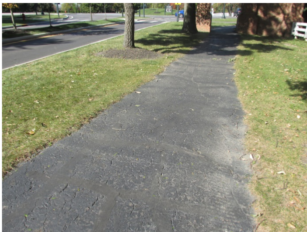
Cracks at asphalt pavement walking path at Lambton Park
