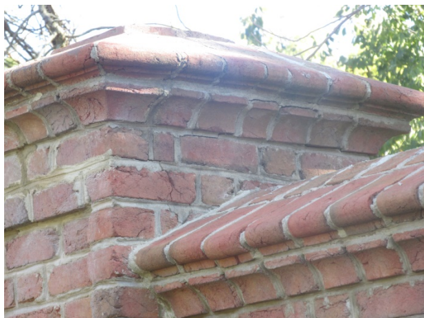
Cracks at masonry monument
