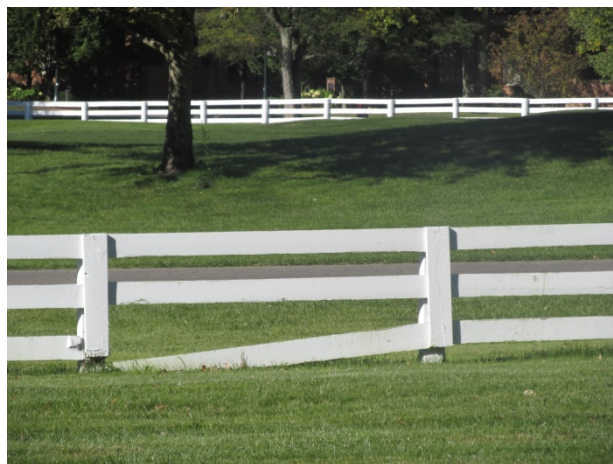
Loose picket at wood fence
