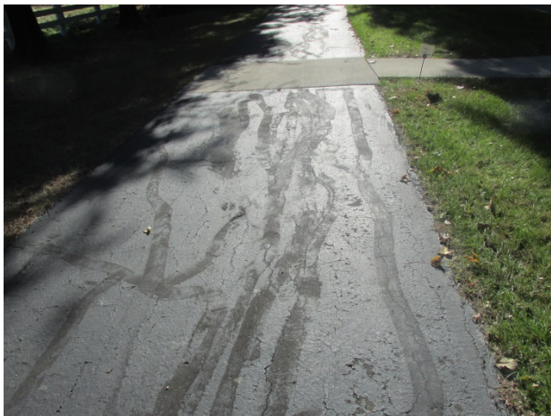
Cracks at asphalt pavement walking path
